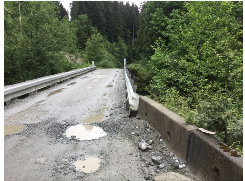
Guard Rail condition at downstream right bank
