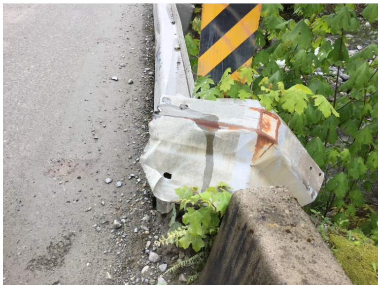
Guardrail damage at upstream left bank
