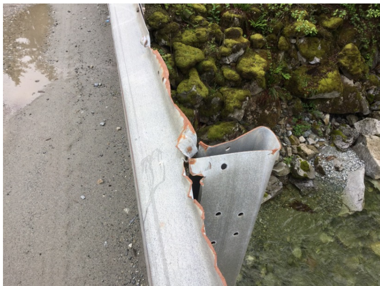
Guard Rail condition at upstream near center span
